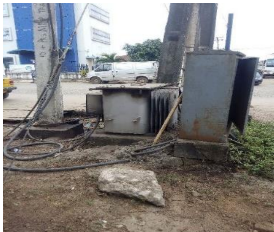
Plate 11: Dilapidated transformer opposite a commercial bank.
